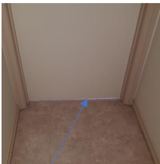
Gap under doors
